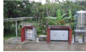
A Trunz solar installation in the Philippines
