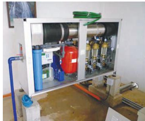
Figure 2: The Trunz Water Box TWB 002 in the Water and Pumping Station
